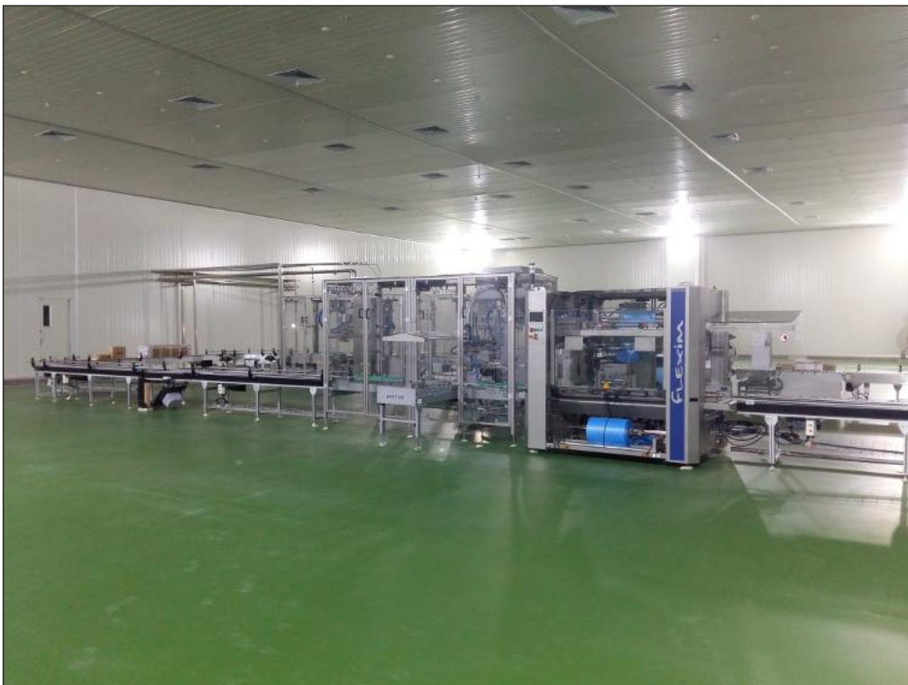
Filling Lines Area (FATS)
