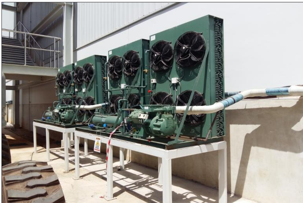
Cold Room Condensor
