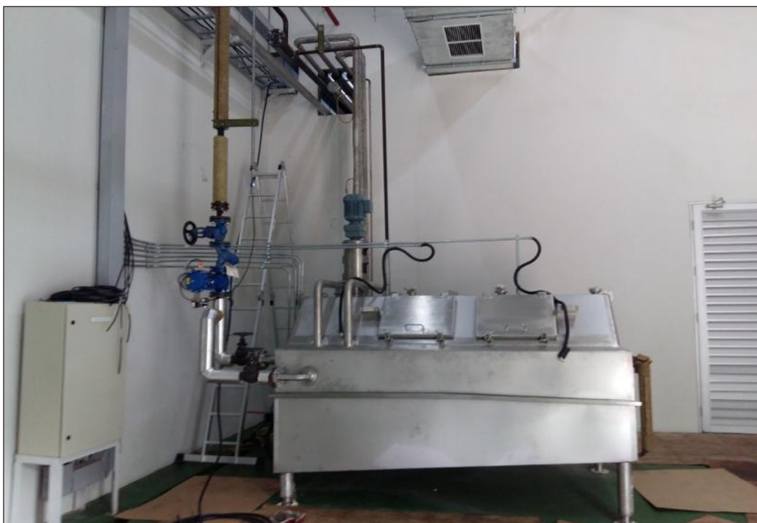
Comp. Air Room (Low Pressure)
