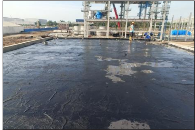
Substation Roof Waterproofing Membrane
