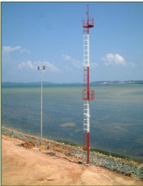
Yard Lightning Protection, External Lighting & CCTV Poles
