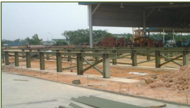
Steel Pipe Rack
