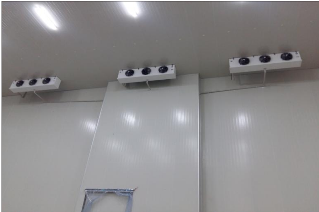
Cool Room Evaporator
