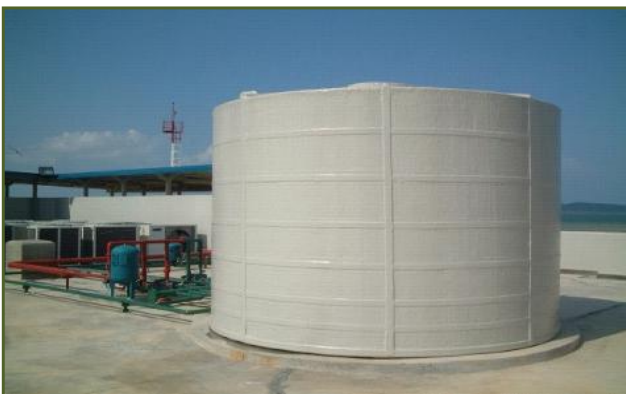
Fiberglass Roof Water Tank & Water Pump
