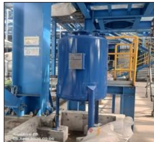
Equipment 3D-751 (Elevation 0.000)
