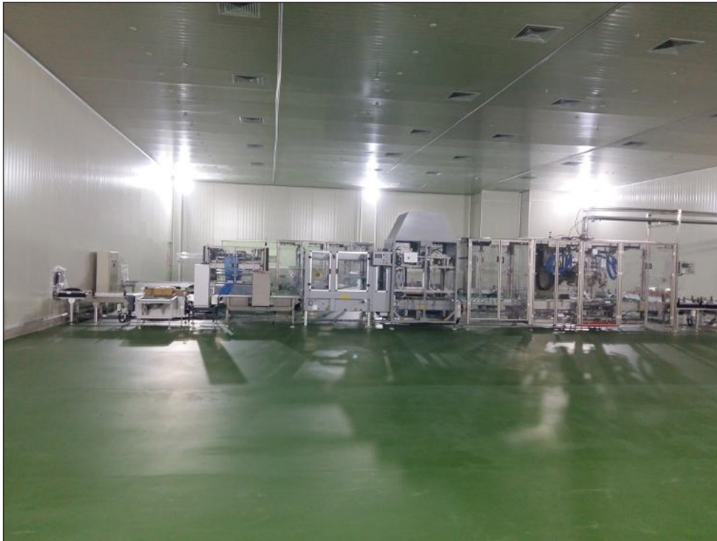
Filling Lines Area (FATS)
