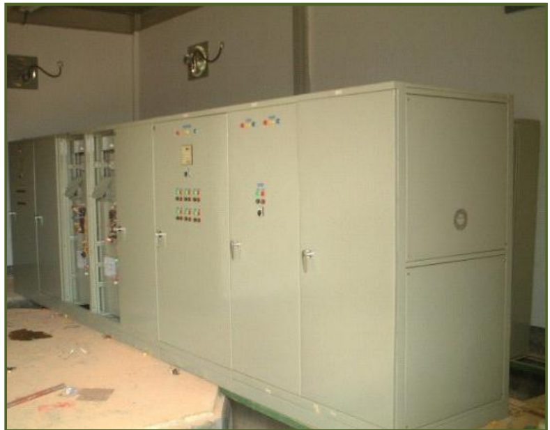
Electrical Main Distribution Box
