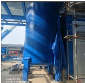
Equipment 3D-762 (Elevation 0.000)
