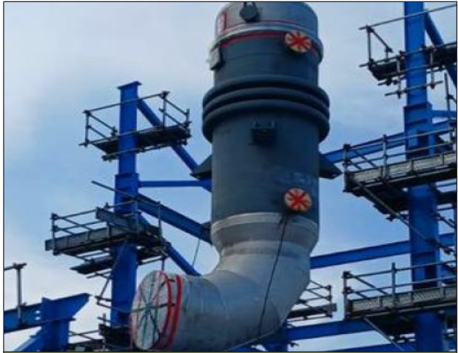
3E-303 (Reboiler) (Elevation +12.000)
