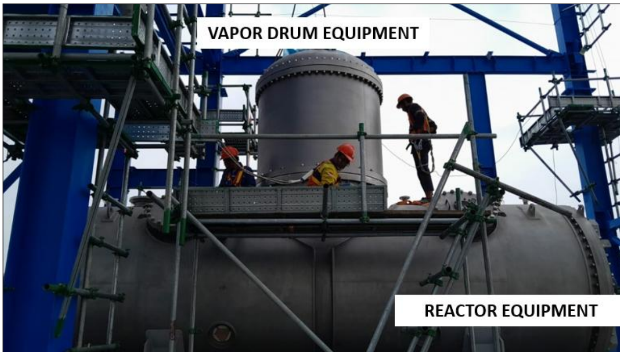
THE VAPOR DRUM EQUIPMENT ALREADY ON PLACE
