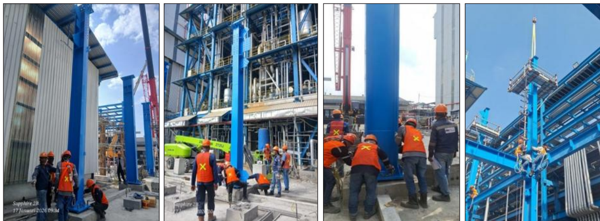
Erection Column Glycerine & Fatty Acid
