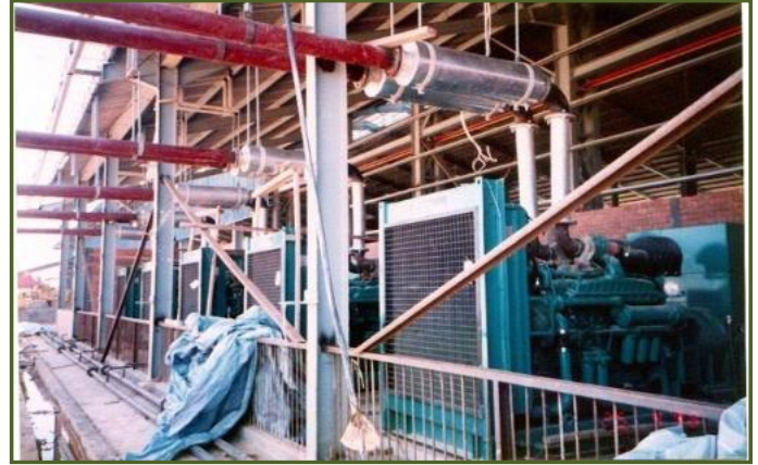
5 Units of 350 KVA Genset
